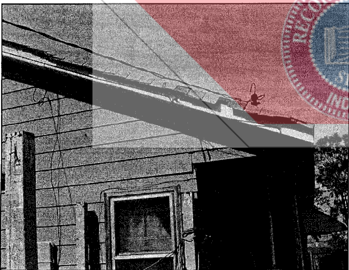
Rear of house, roofing older & shows some patchwork
