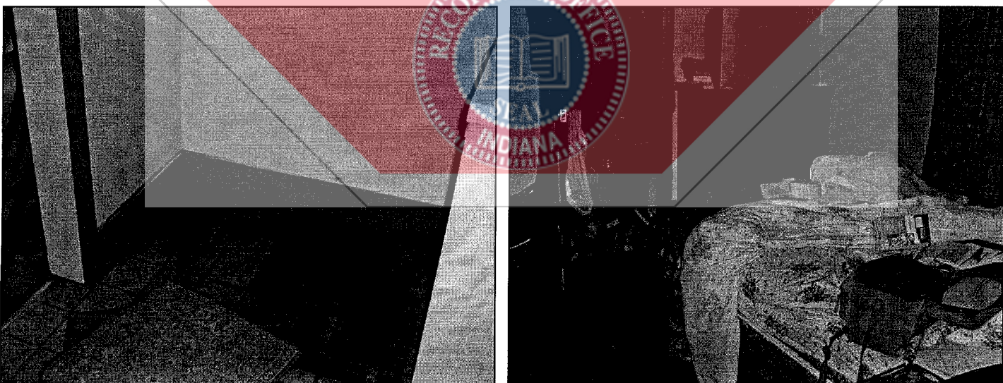
Interior-kitchen floor damaged
