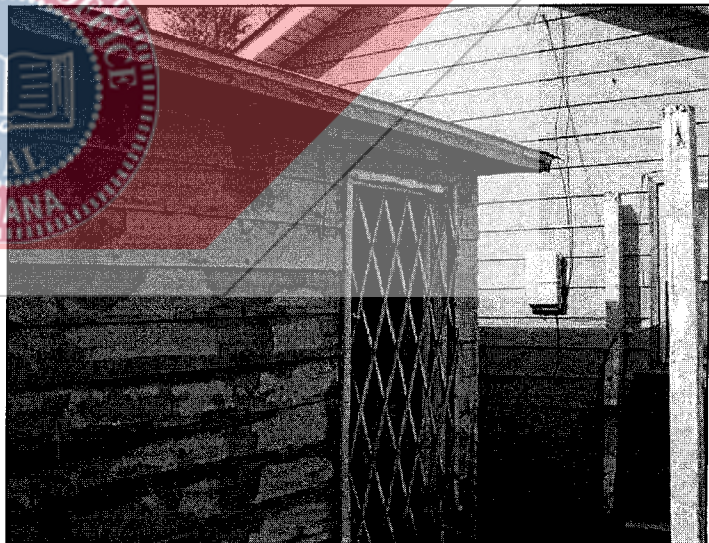
Rear of house & side of garage (peeling paint on garage, door needs repair)
