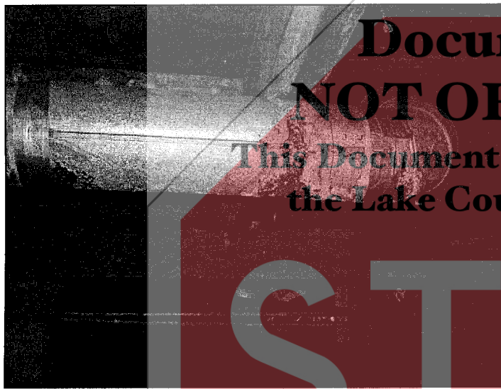
Interior-some rust noted on heating pipes in basement
