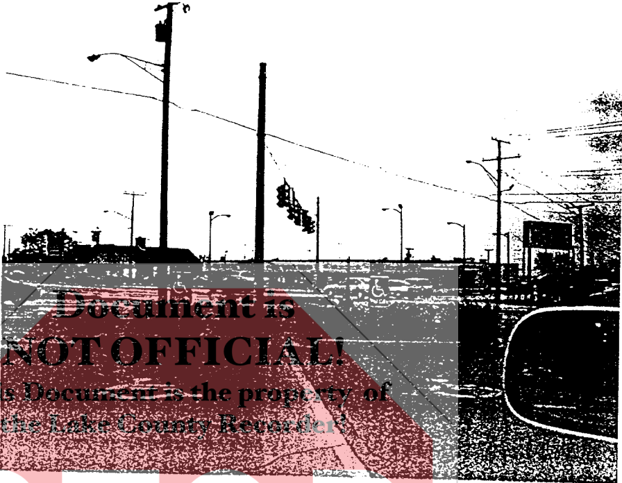
CRACKS IN PARKING LOT
